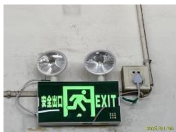
Safety exit sign and emergency light.JPG
